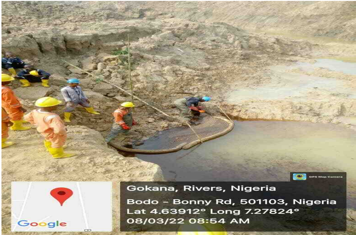
Containment and recovery of free phase crude Plate 3.44: Excavated trench with free phase crude oil
