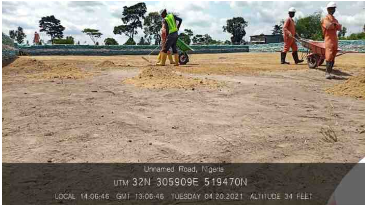
Stabilizing the floor after grading and sloping prior to the installation of HDPE Liner
