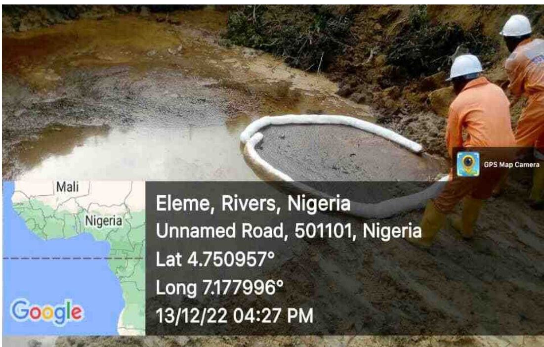
Containment of crude oil
